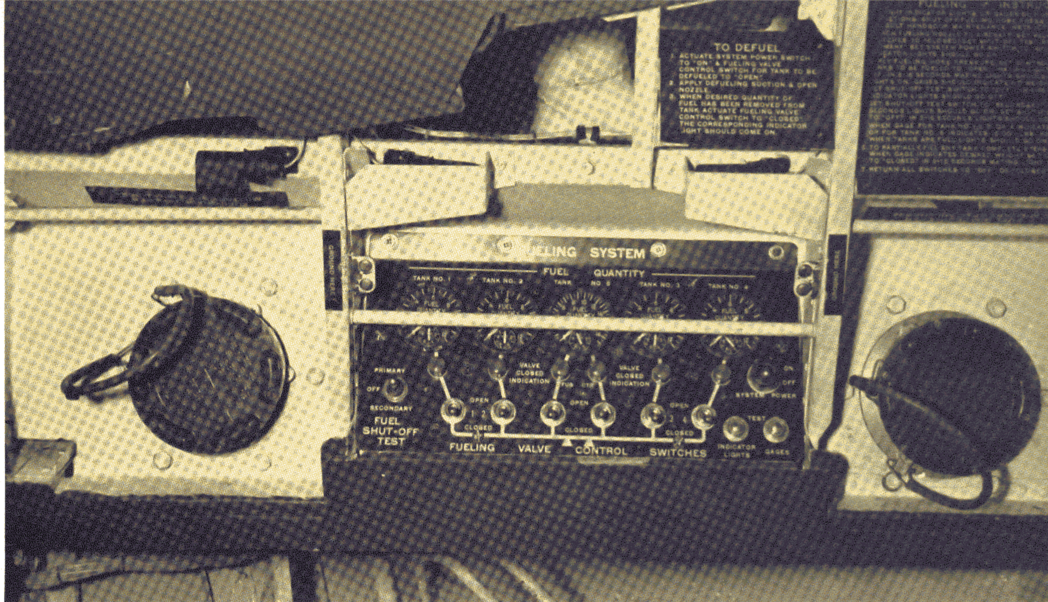
Figure 7 Fueling Control Panel
