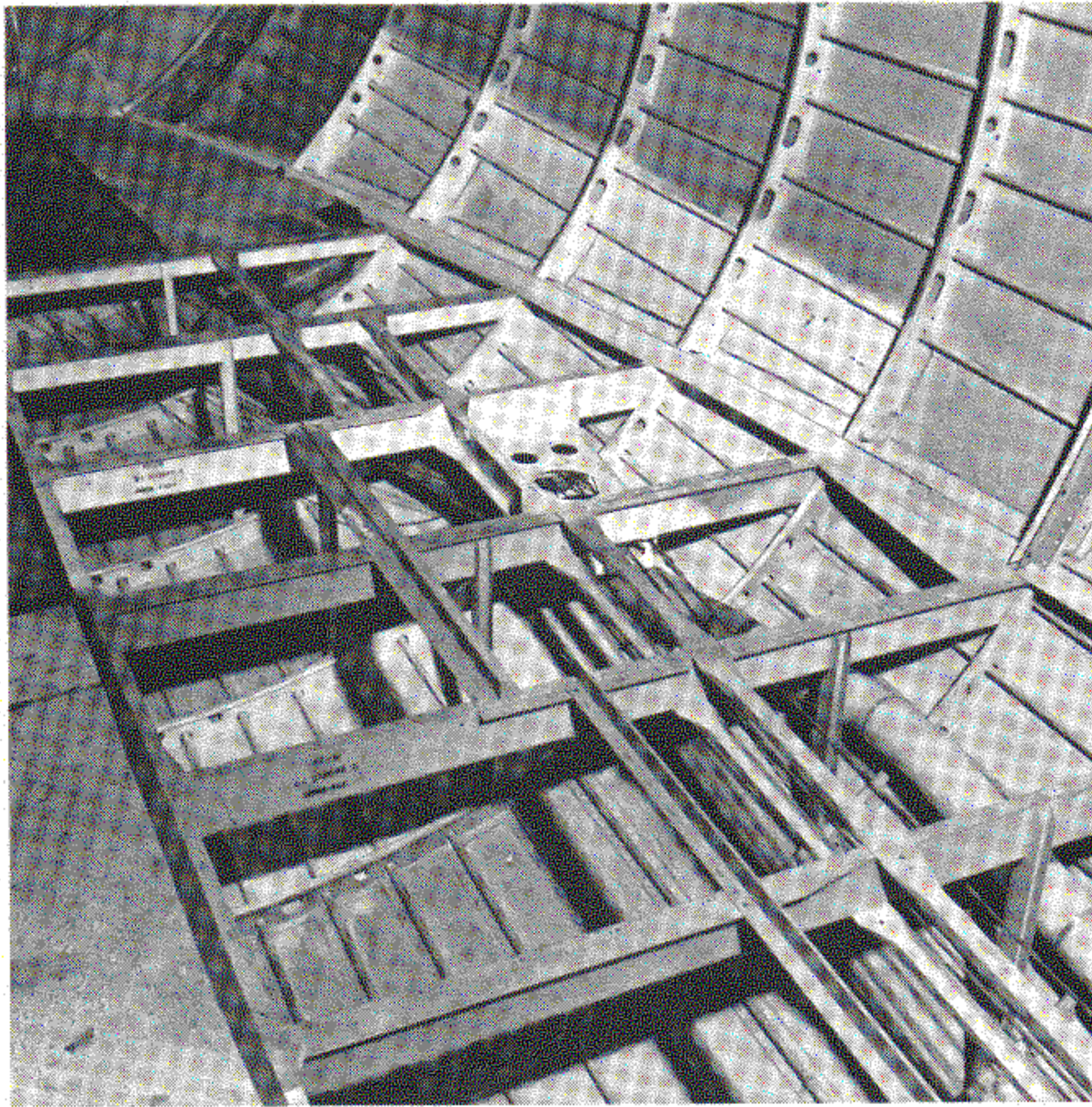
Figure 16a Structure in Galley Area Protected by Acid-resistant Lacquer
